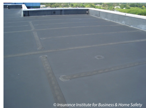
Single-ply EPDM membrane roof cover (mechanically attached).
