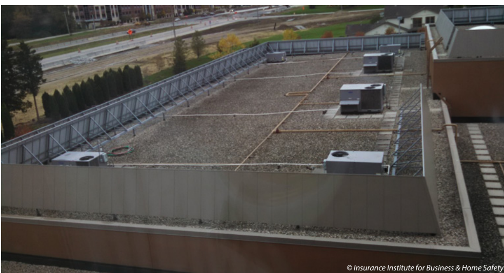
A wind screen on a low-sloped ballasted roof concealing rooftop equipment from the street and neighboring buildings.
