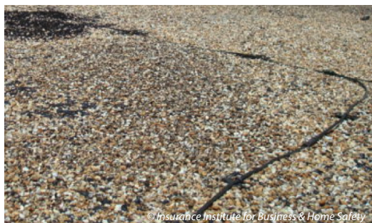
Built-up roof cover with gravel embedded in asphalt. (A lightning protection cable also is shown.)
