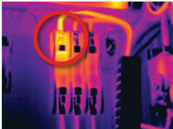
Shown above is an example of what a hand-held thermal scanner could show you, with a potential hot spot circled.
